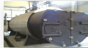
Waste Heat Recovery Boiler 2 TPH at AP-4 Line
