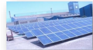
4.8 MW Solar Plant
